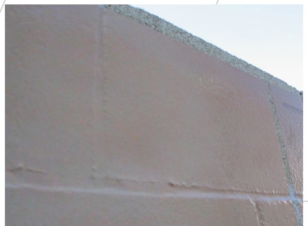
Figure 4: Example of bad install with popped graphics in grout.
